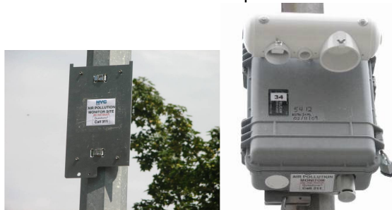
Fig. 3. NYCCAS pre-installed mounting plate and NYCCAS air sampling unit mounted on lamp-post.
